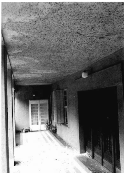
Fig. 24 Damages on the entrance of the Observatory main building after the bombardment of Zvezdara suburb by NATO agresors on 31 st May 1999 between 3 h 45 m and 4 h 05 m in the morning.
